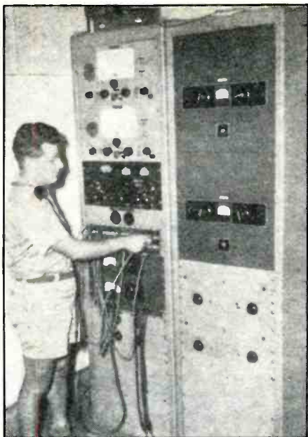
The Spindle Eye's main patch panel in the broadcast control room. The technician is adjusting the compression amplifier. The dark radio midway up the rack is a Hallcrafters S-36 monitor receiver.
